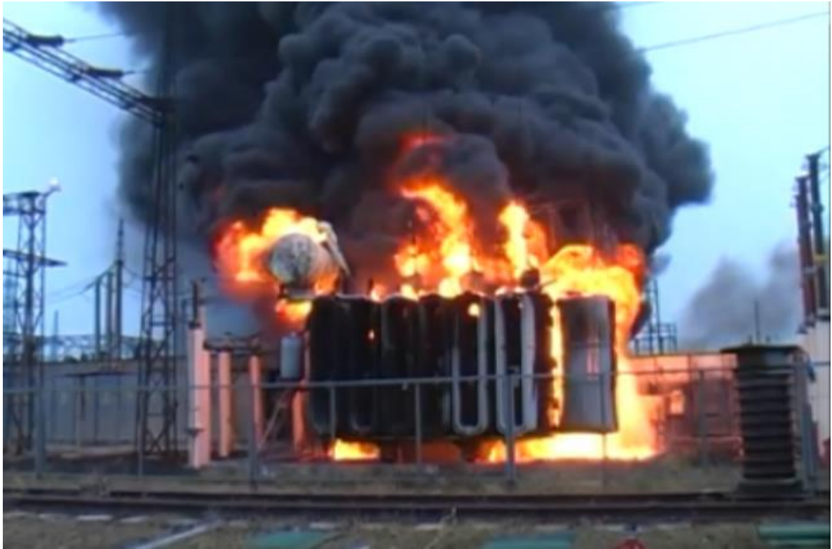
Figure 2. Transformer on fire.
