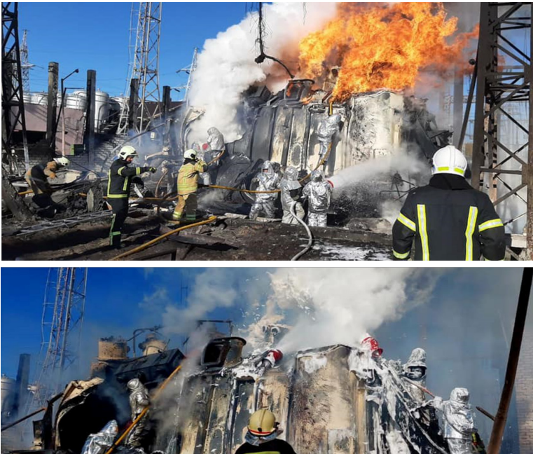
Fig. 2.7. Extinguishing a fire in a group of transformers as a result of shelling
