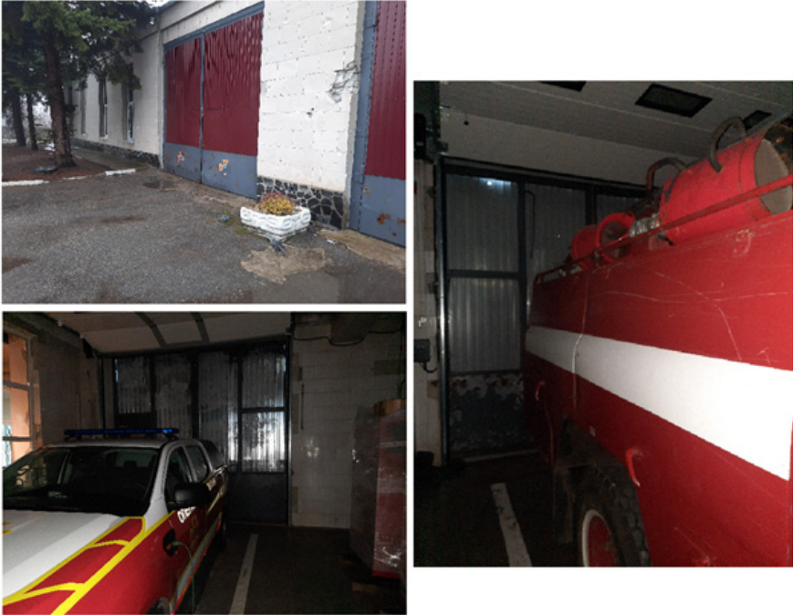
Fig. 6.7. The condition of the gate after the shelling of the surrounding area (the glass was replaced by corrugated board). Examples of placement of operational vehicles with the rear to the side of the gate
