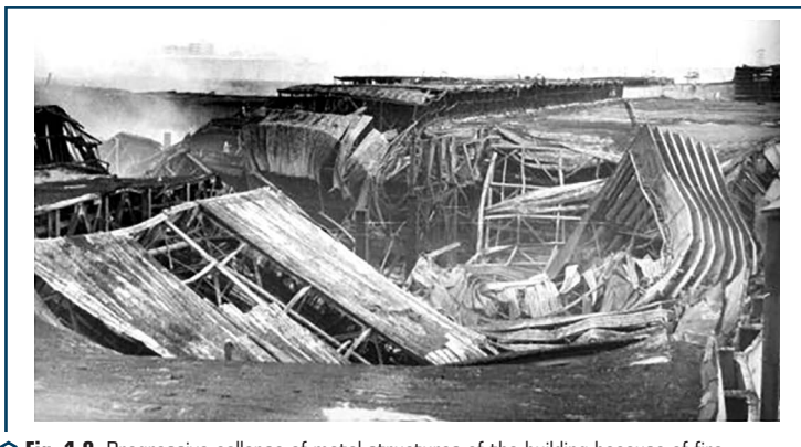
○ Fig. 1.8 Progressive collapse of metal structures of the building because of fire
